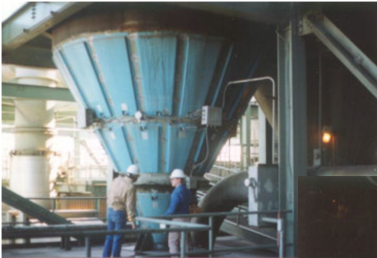
← COAL SILO HEATED WITH FRP HEATING PANELS AT A MAJOR UTILITY IN THE NORTH EAST, USA
